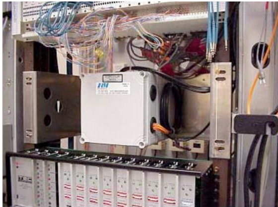
5-CARD SHELF INSTALLED IN MOUNTING BRACKET
