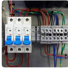
Terminal Blocks & Breakers
