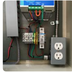
AC Power Outlets
