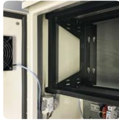
Equipment Rack Rails
