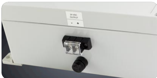
Battery Pack Terminals and fuse
