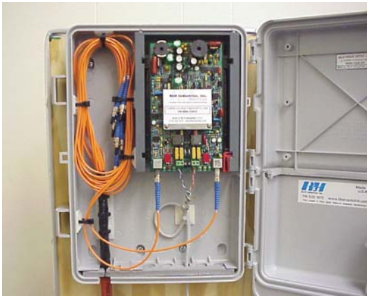
Figure 4-1 RLH HDSL1 Adtran CO Card installed inside RLH card housing
